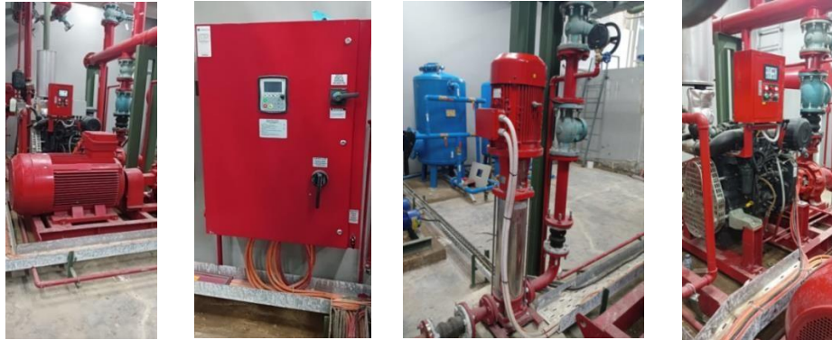
Gambar 4.9 Pompa Fire (Electric Pump & Diesel Pump)
