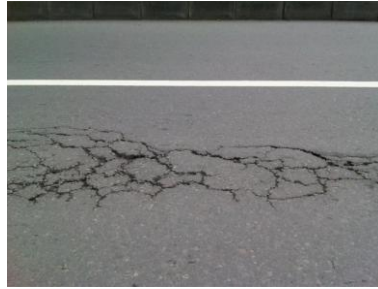
Gambar 2.2 Retak Rambut (Hair Cracks)
